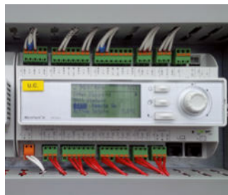
Controller box upgrade
